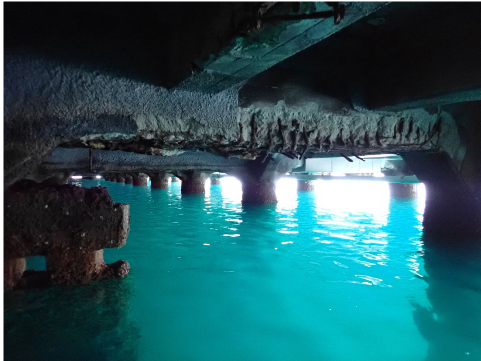
Photo 4: Typical Girder Spall
