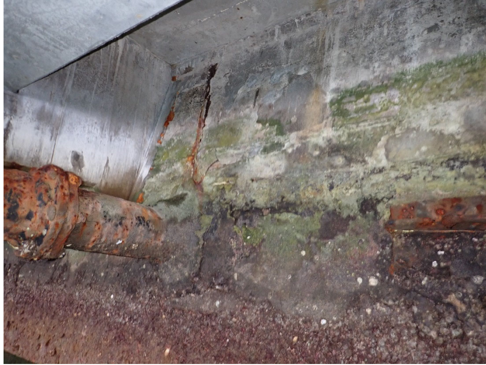
Photo 5: Typical Vertical Spall
