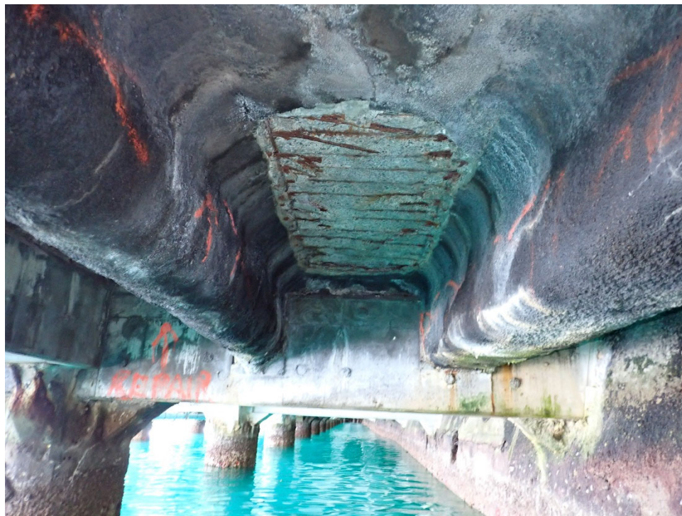
Photo 2: Typical Slab Spall
